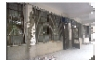
Shear failures in short "active" columns
